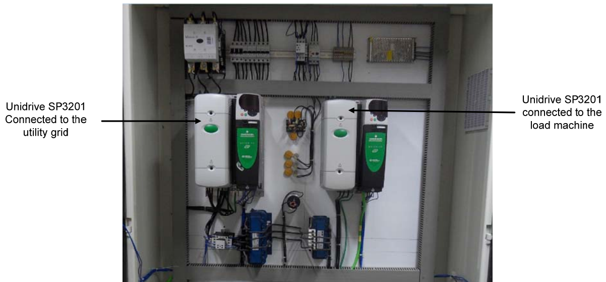
Figure 10. DC/AC converters (Unidrives) used to drive the load machine.
